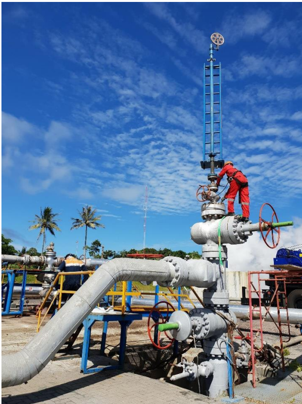
Figure 3: Typical geothermal well – well head
